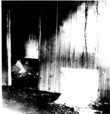
Scenes from inside a St. Georges home located on Annette Ave. that was completely destroyed inside by fire. The local fire department worked for almost five hours to extinguish the blaze and clean up the mess.
