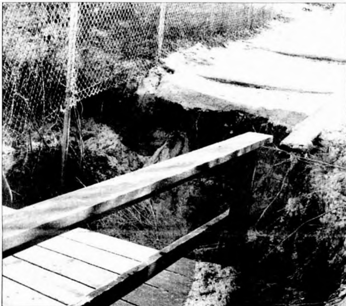
Lester Beach Walkway undercut by last week's storm. All stairways to the beach were damaged.
