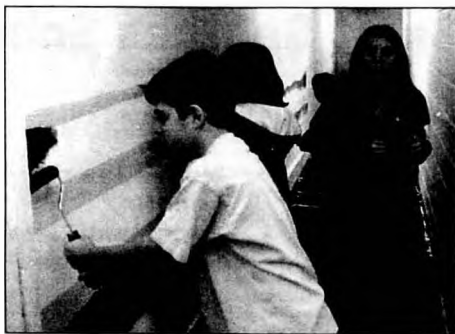
Powerview School students participate in Project K.I.N.D. This part of their project was to help with the Powerview Arena. Students painted the lower level of the arena.
