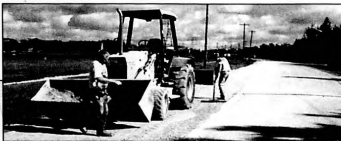
Maple Leaf Construction unloads (above) and levels (top right) fill in the process of widening McArthur Avenue five feet, from Minnawa to Oak Street
